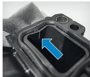
Fig. 2: Breakage (damage pattern)
